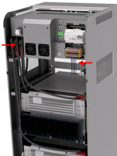
Figure 27 – cables obstructing the cassette input
